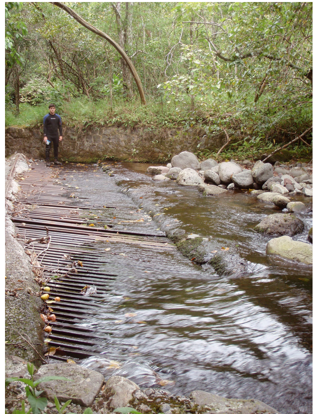
Fig. 2. Water capture at a diversion inlet in upper Waihee Stream, Maui, Hawaii
